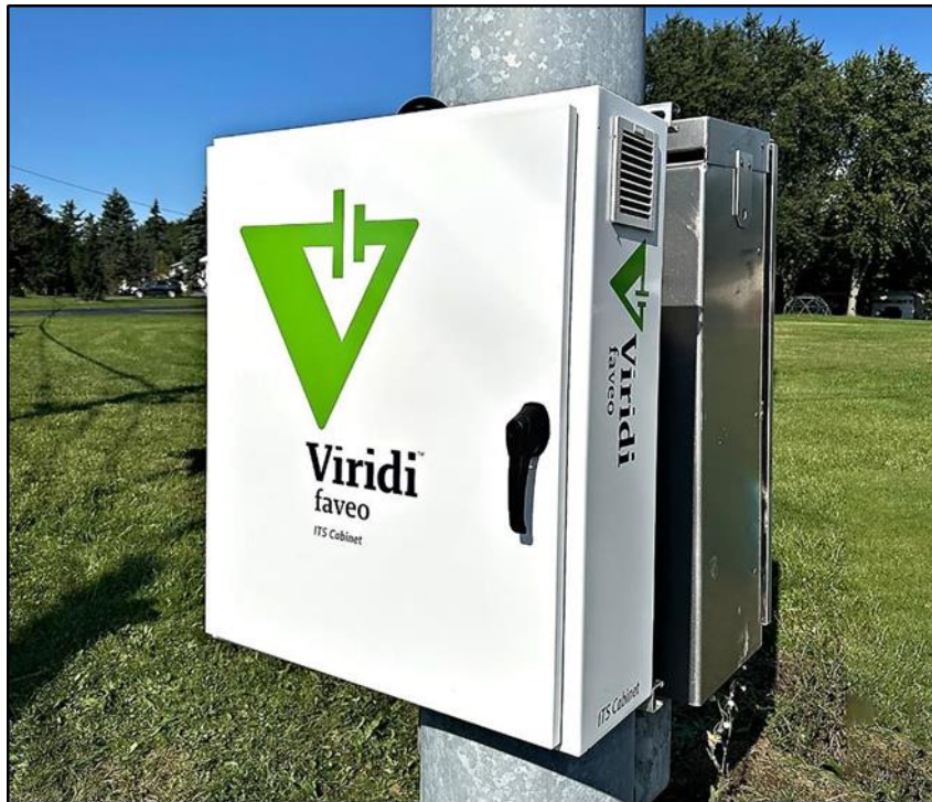
Faveo Installation in Lancaster, New York
