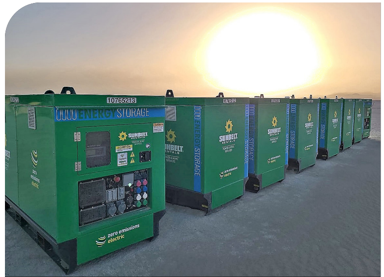
RPS150 portable energy storage units using Viridi technology help power the Burning Man event in Black Rock City, NV.
