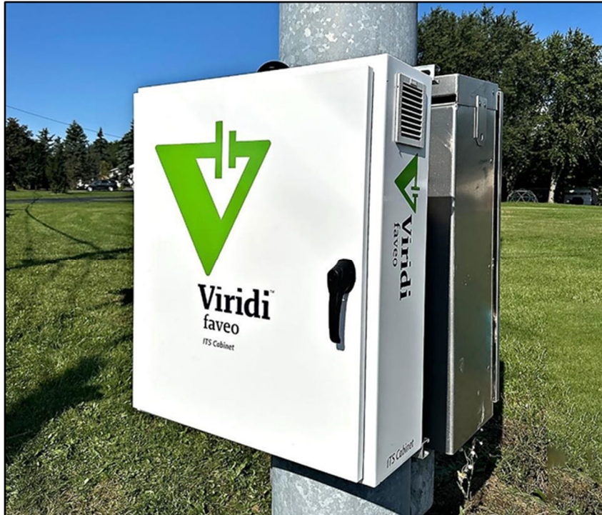
Faveo Installation in Lancaster, New York
