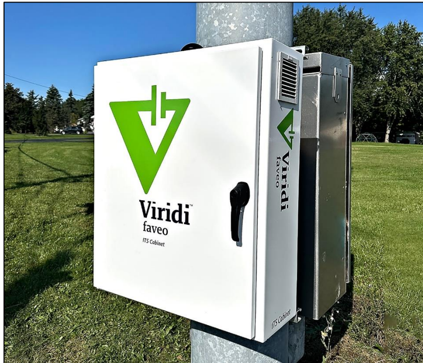
faveo installation in Lancaster, NY
