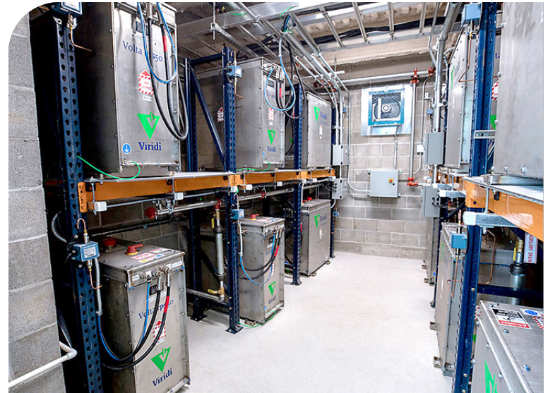
Twelve RPS50 lithium-ion batteries installed in a dedicated room at HWI. No incremental cooling, ventilation, or fire suppression is needed with Viridi BESS (those seen in the photo were pre-existing and were not removed).
