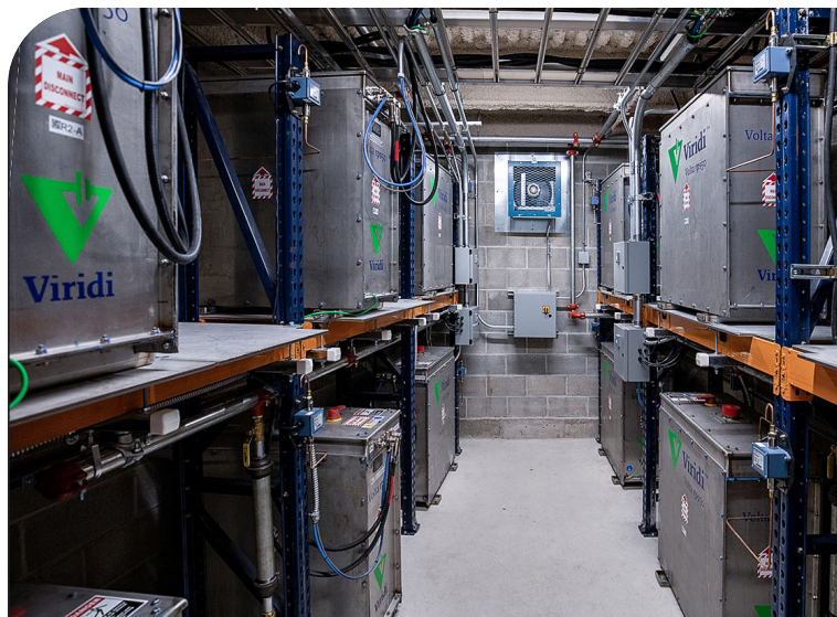
Twelve RPS 50 lithium-ion batteries installed in a dedicated room at HWI.
